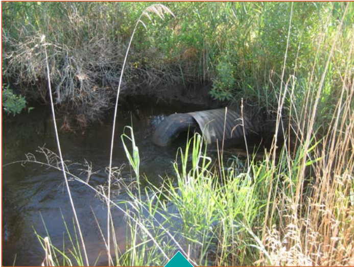
Deal Island Road Existing Culvert with rubber tire jam
