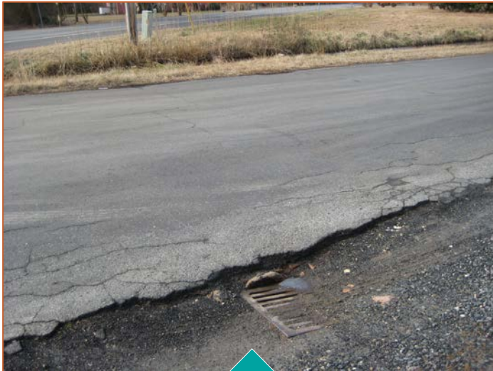
Hodson White Road Clogged grate inlet and culvert at Deal Island Road intersection
