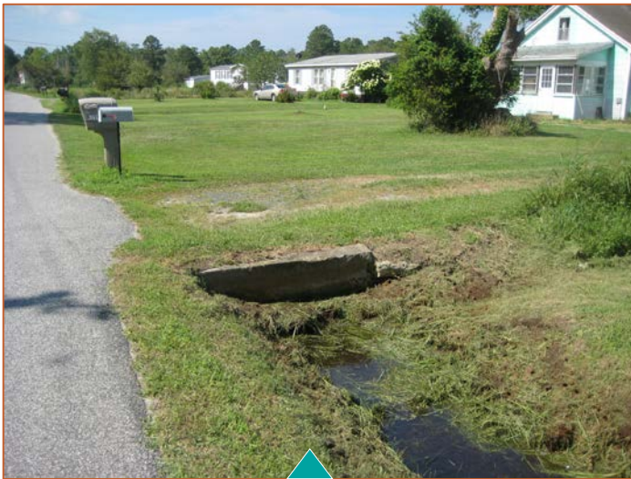
Champ Road Submerged and partially clogged culvert (10260 Champ Road)
