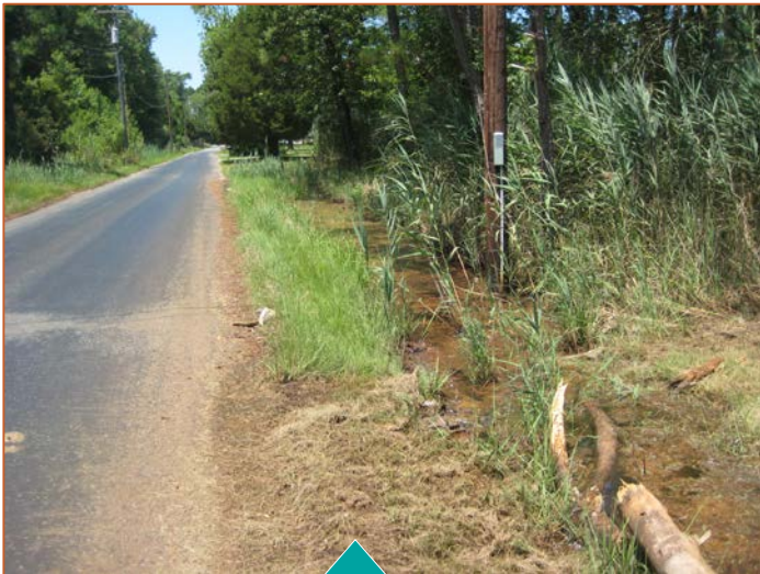
Hodson White Road 18" RCP Culvert crossing into the Deal Island Road crossing ditch
