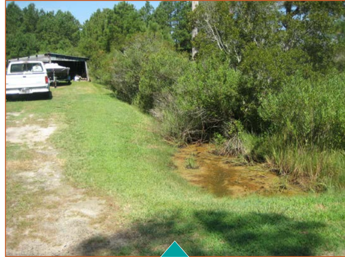
Champ Road Standing/stagnant water at non-roadside ditch
