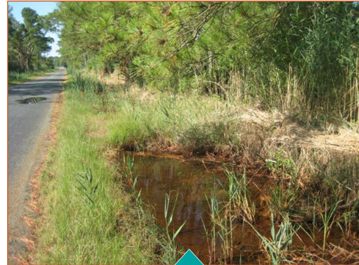
Long Point Road Standing water and vegetative blockage
